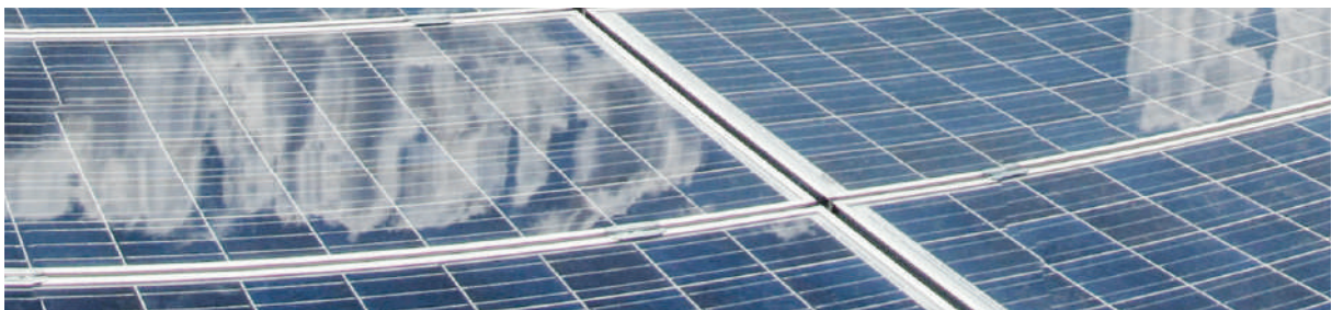
Photovoltaic panels installed on the headquarters roof
